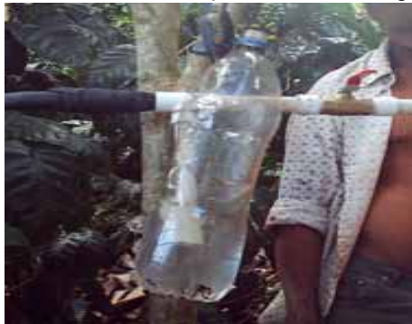
Above: Pressure release valve secured to a tree.
